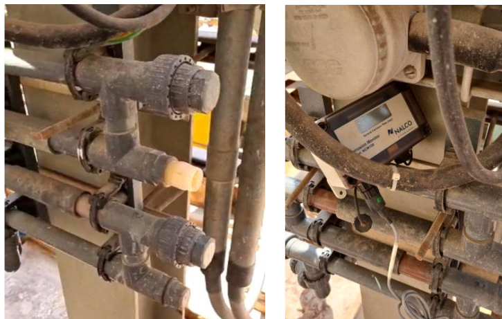
Figure 3. Left: coupon sample location on rack, Right: PVC rack with NCM monitor attached to corrosion probe.
